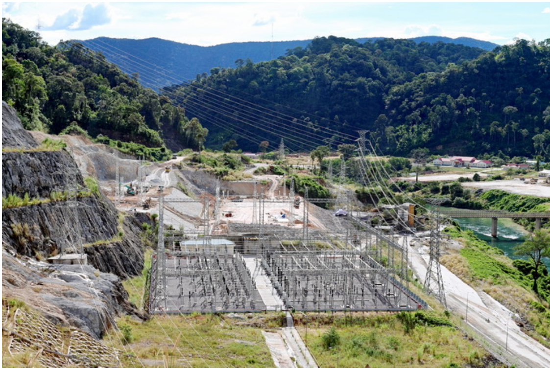
230kV switchyard and 230kV line from Xekaman 1 to Pleiku 2, Vietnam
