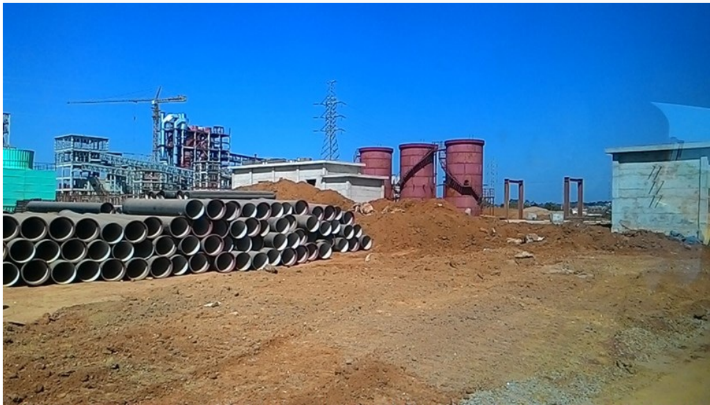
The construction site of Vietnam's second bauxite refinery plant in the central highlands province of Dak Nong. Photo: Manh Quan
