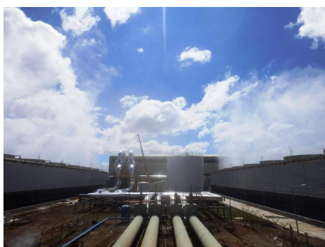
Olkaria I Geothermal Power Plant
