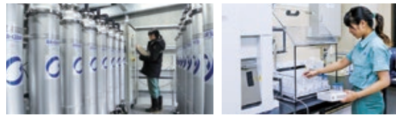
Membrane treatment plant delivered to a seafood processing factory
