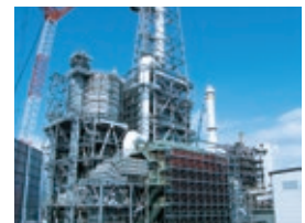
Biomass boiler, Oji Materia Fuji Mill
