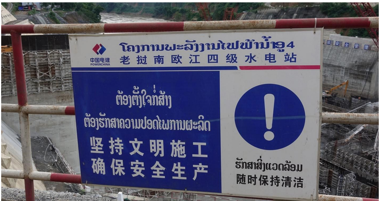
The Nam Ou 4 dam, currently under construction. Khua district, Phongsaly province. Oct 2018 (photo by author)
