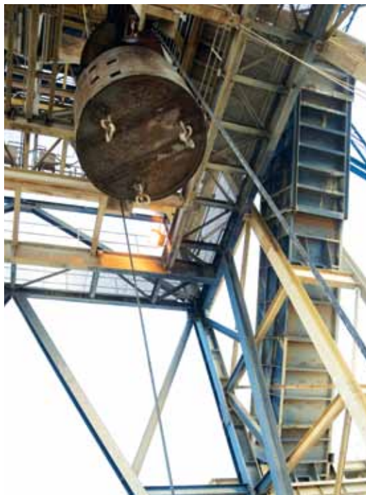
With the 'owner's team' in charge, Kibali achieved a sinking rate for the vertical shaft 50% higher than the industry norm, reaching the bottom at 751 metres three months ahead of schedule.
