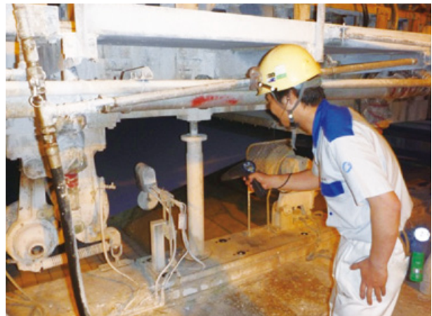
Investigation of compressed air leakage (Oji Paper Yonago Mill)
