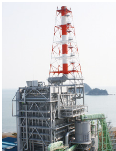
Tomioka Mill's biomass boiler
