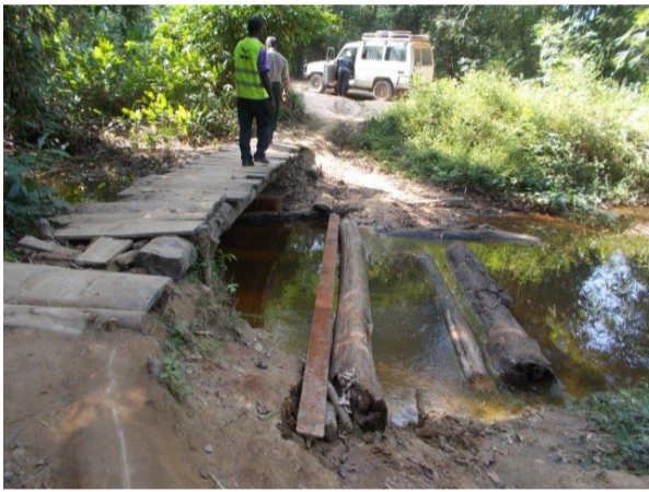
Delivery of materials for bridge repairs to Bahn Town and Yolo Town
