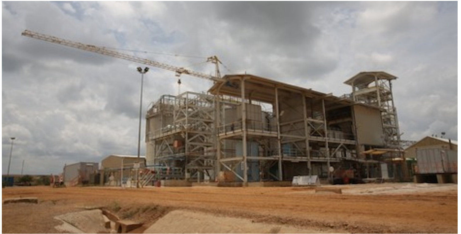
Image of the Youga plant, courtesy of Endeavour Mining.
