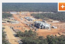
Kansanshi and Sentinel mines will use the same smelter, which is currently under construction.
