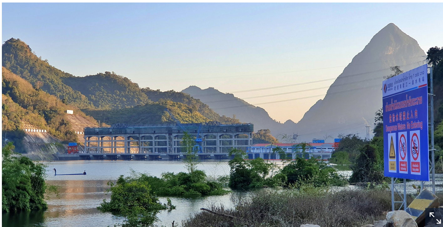
The Nam Ou 1 dam, still under construction, has flooded Lat Tha Hae's riverside gardens (Image: Ton Ka/China Dialogue)
