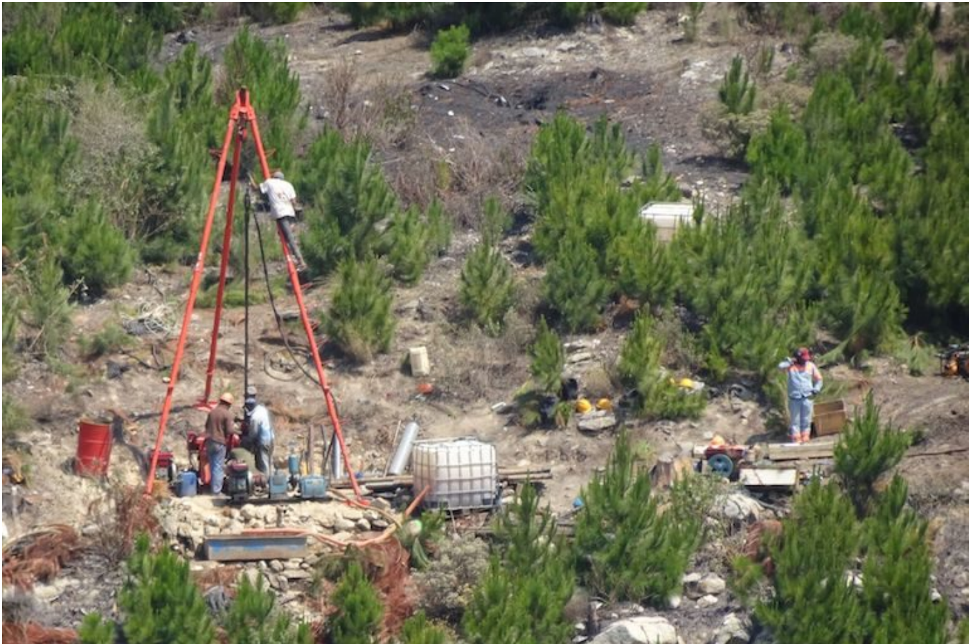
Tozzi Green workers perform core drilling at the proposed dam site near Farihitsara. Image by Mihary Velo Soa and Tiana Andria, MALINA network, Transparency International – Initiative Madagascar.
