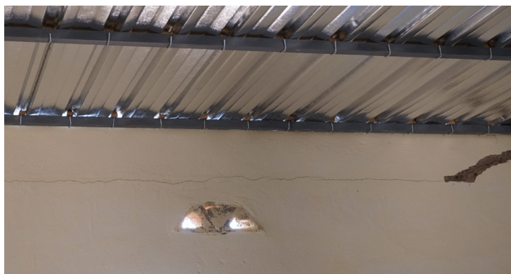
Cracks in the wall of a newly constructed house for resettlement in the new Bouly village (Photo: Merle Groneweg, 2017)
