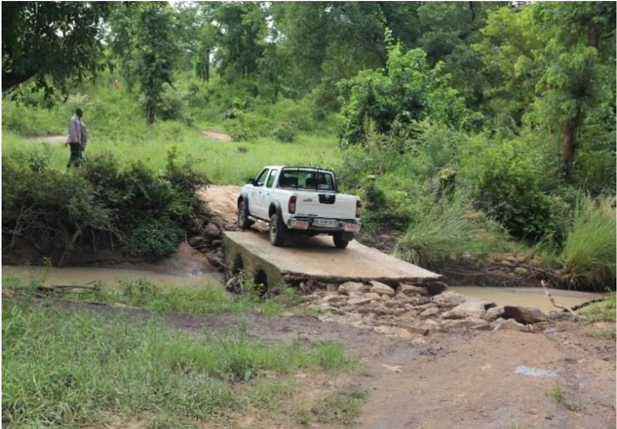
Fig. 30: Joint Head Office and Tumu Forest District monitoring team crossing a dilapidated bridge near Tanvielle
