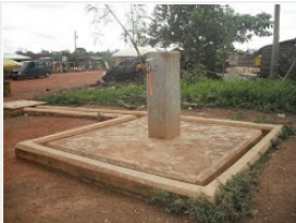
A standpipe for a rural community
