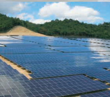
Solar power generating system delivered to Taihan Techren Co., Ltd. by Sojitz Pla-Net Corporation
