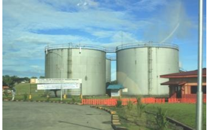
Figure 150: Storage tanks for CPO
