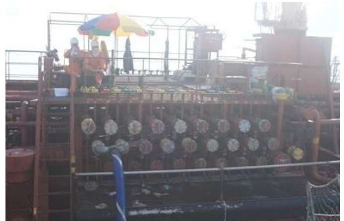
Figure 160: Pipes to load palm oil into the tanker
