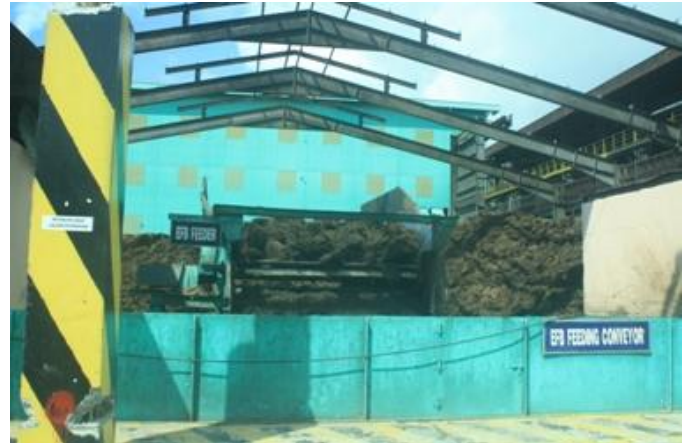
Figure 156: Biomass plant in Sahabat to generate electricity
