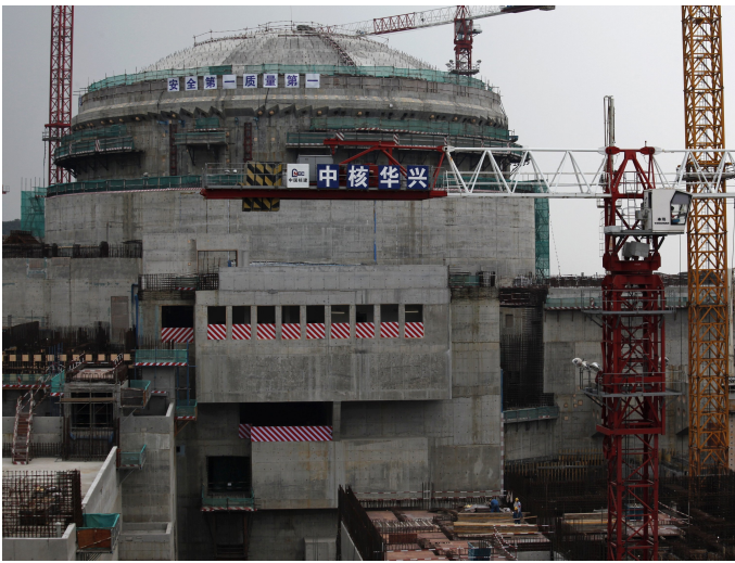
Workers (bottom) stand in front of a nuclear reactor as part of the Taishan Nuclear Power Plant seen under construction in Taishan, Guangdong province, on October 17, 2013 Bobby Yip/Reuters
