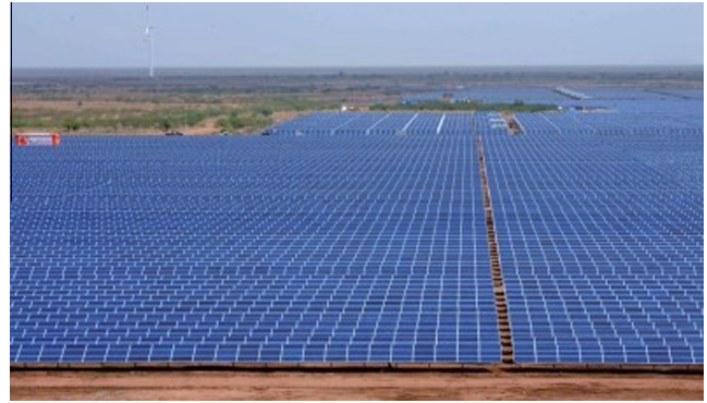
Fig. 1. A view of Charanka Solar Park, Gujarat. Source: first author.
