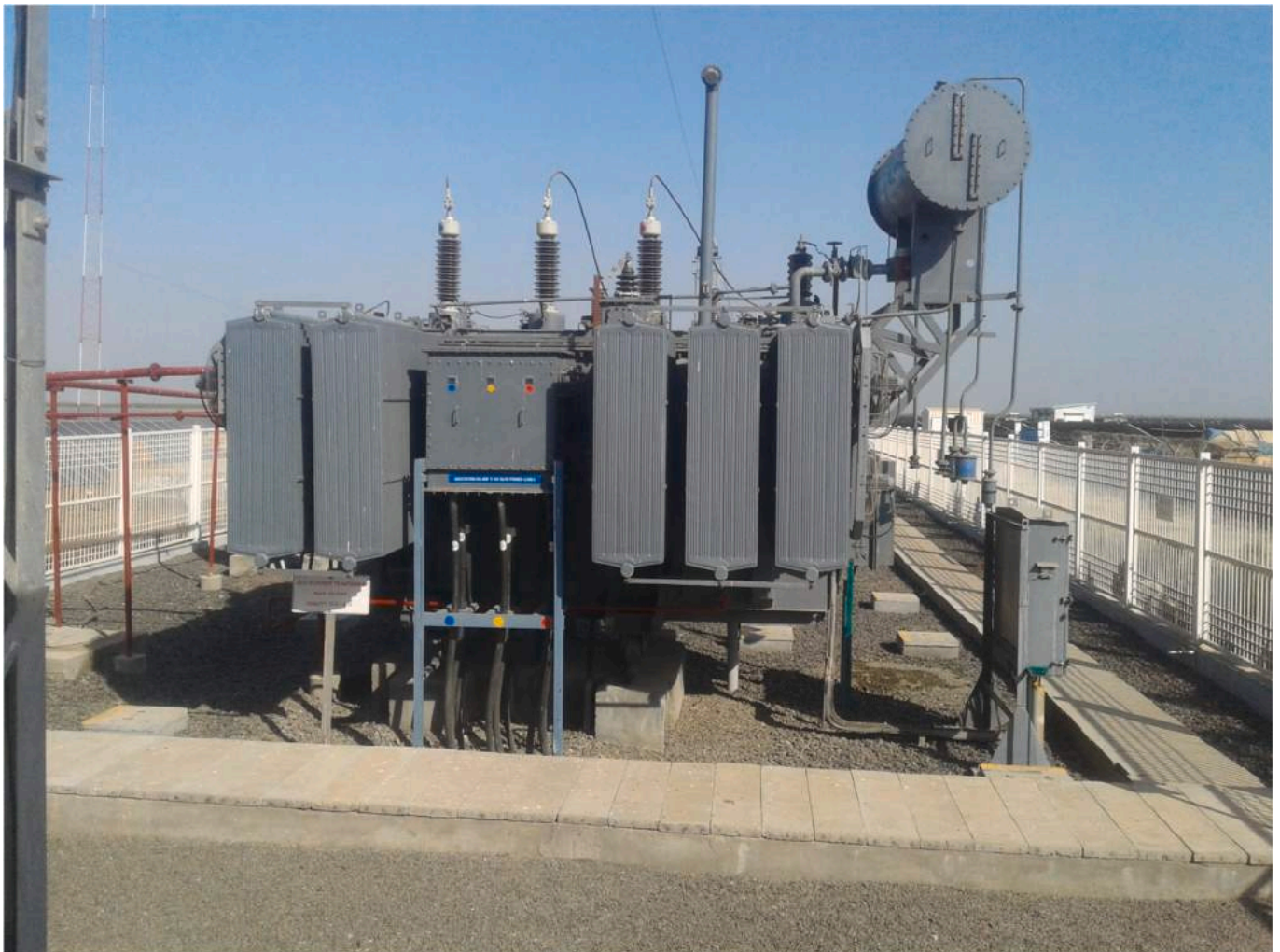
Fig. 3. Substation transformer at Gujarat Solar Park. (Photo: Ryan Stock).
