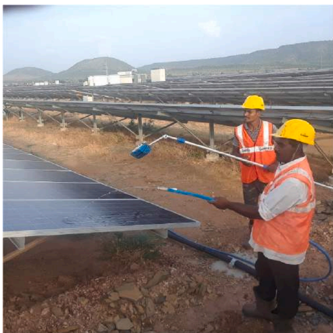
Fig. 4. Laborers washing solar arrays at the Kurnool Solar Park. (Photo: Ryan Stock).
