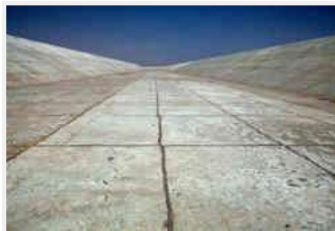
An empty water canal at Sheikh Zayed, near Toshka (Photo: NPR)
