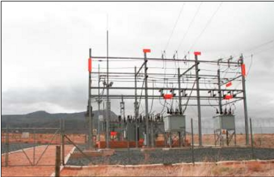
Figure A.5.2: A typical electrical substation 8 .
