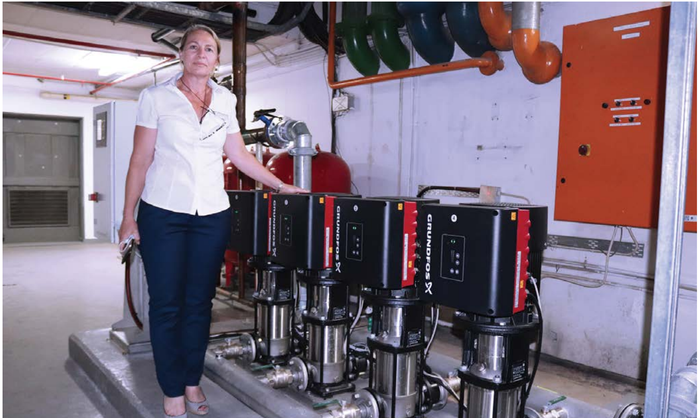
Charmaine Spasojevic, Chief Engineer at the Hilton Hotel, in front of the Grundfos booster pump installation.
