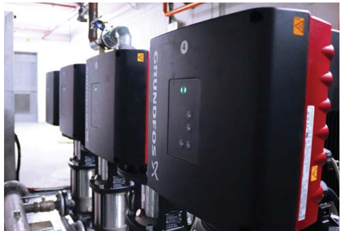
Constant pressure is assured through continuous adjustment of the speed of the pumps.
