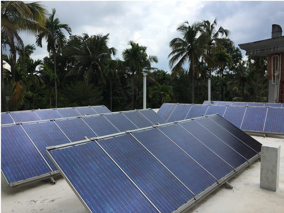
Figure 5. Rooftop solar in Kerala.
