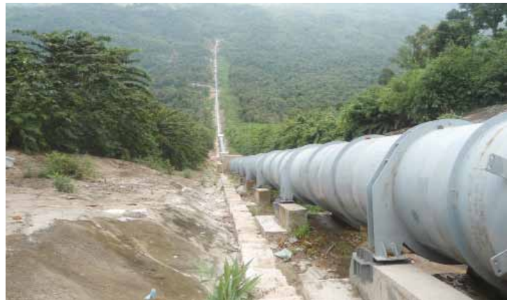
A pipe snakes across the hills of Xekong province, part of the Houay Lamphan Gnai hydro plant.
