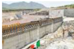
Construction work underway on the Grand Ethiopian Renaissance Dam. Image courtesy of Salini
