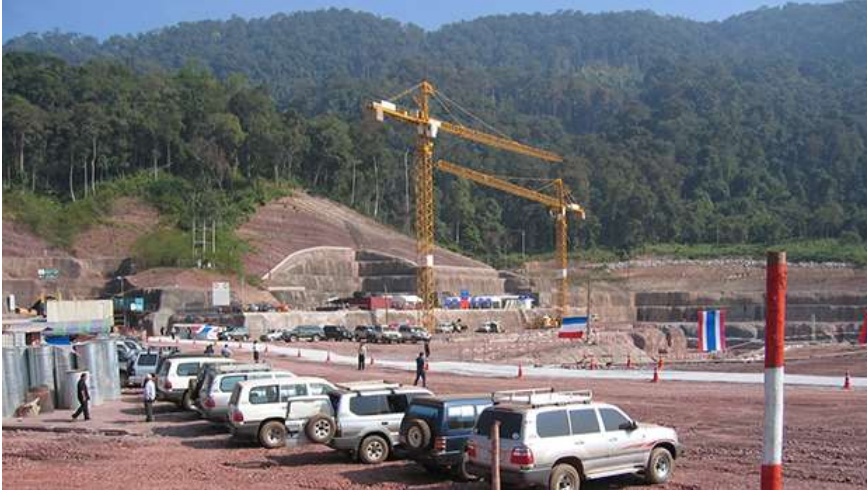
The site of the Nam Theun 1 dam project, in a file photo. RFA Photo
