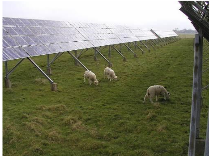
Figure 3.10: PV ground mounted system 20
