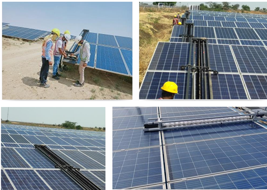
Robotic Dry-Cleaning System Installed at Sites
