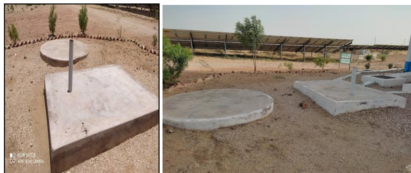
Figure 17: Sample Photographs of Septic Tank at Site
