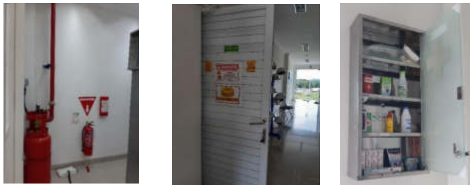
Figure 11 – Safety equipment at the site
