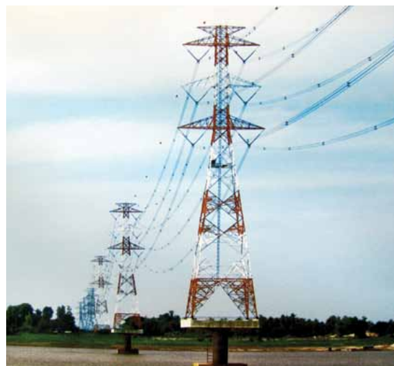
Mekong 500kV transmission lines link electricity supplies between Laos and Thailand.
