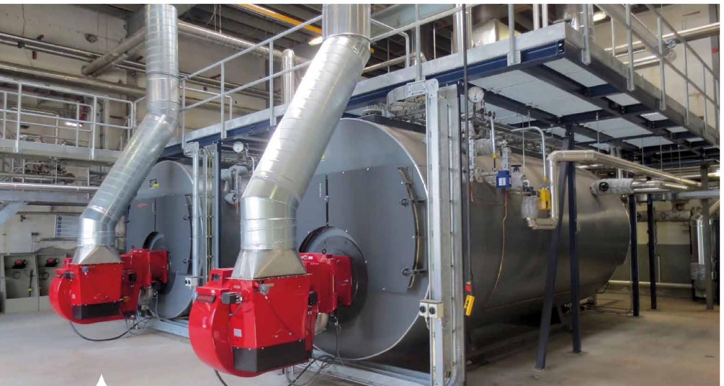
New boilers at KLK Kolb Specialties BV, Delden, Netherlands
