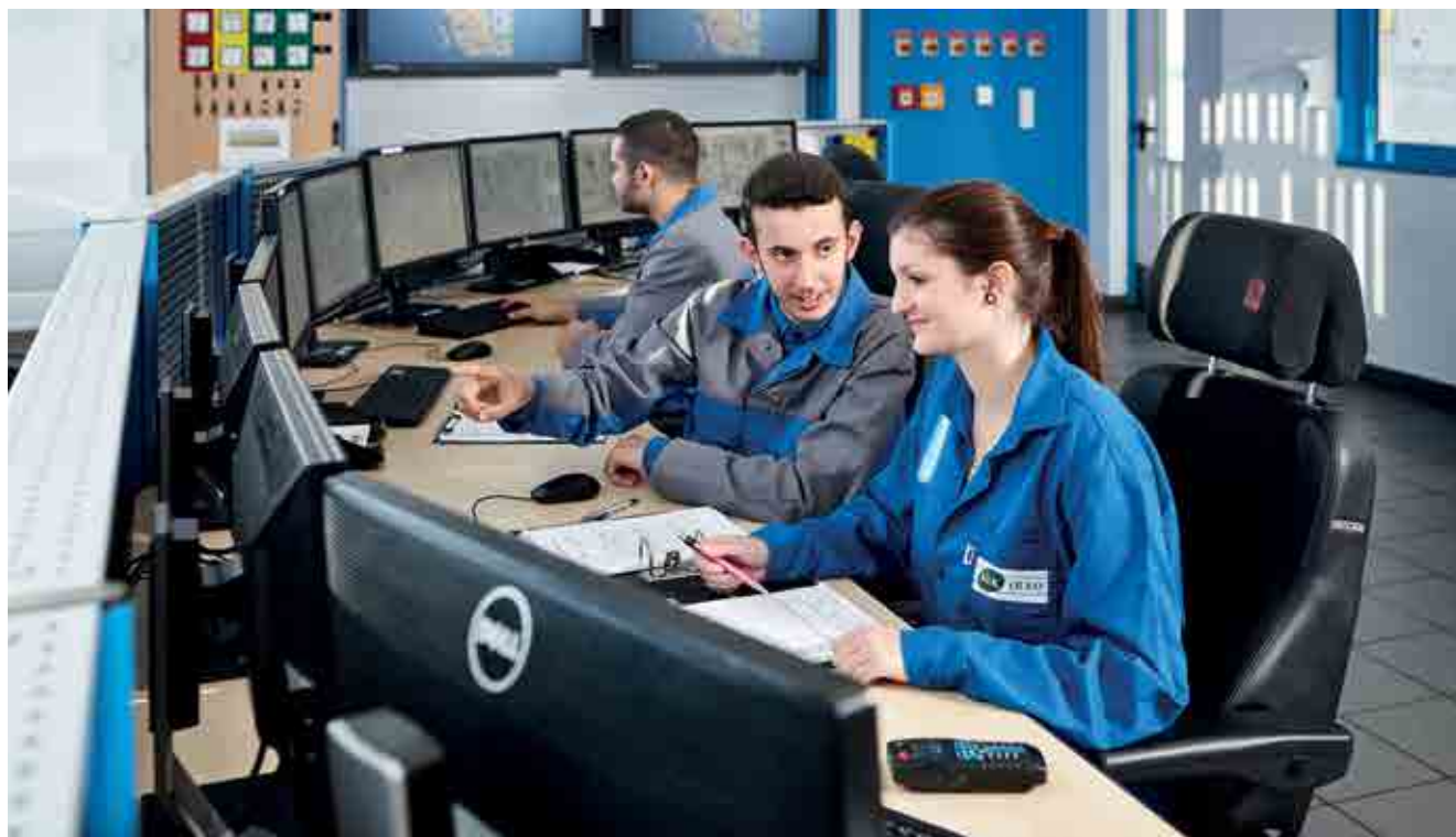
Central control room at KLK Emmerich, Dusseldorf site, Germany
